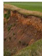
EAOW Intertidal North W2 - coastal erosion 3
