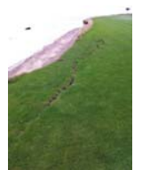
EAOW Intertidal North W2 - coastal erosion 4
