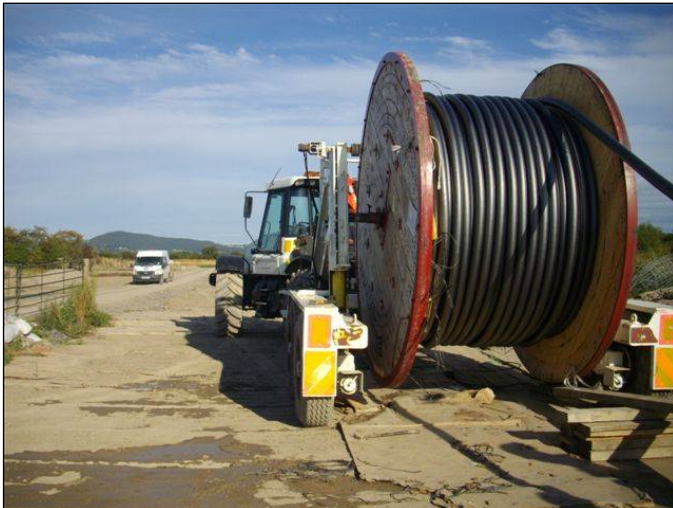
Plate 1: Typical tractor and trailer set up for cable drum transportation (Photo courtesy of Prysmian Group)
