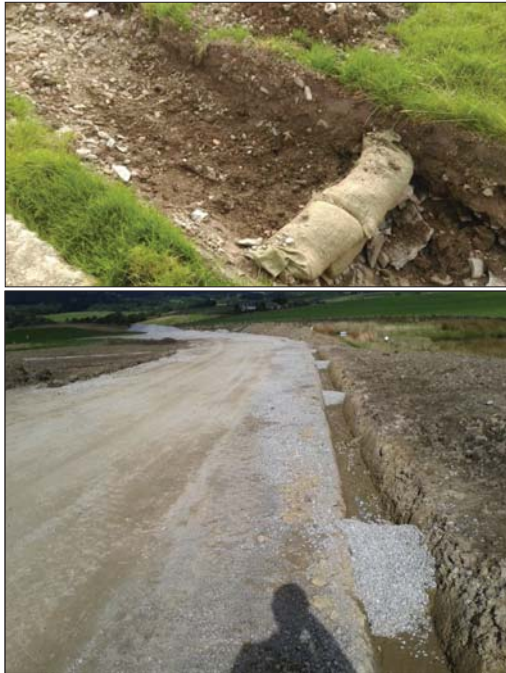
Plate 4: Typical check dams - to be installed in drainage ditches adjacent to the access track
