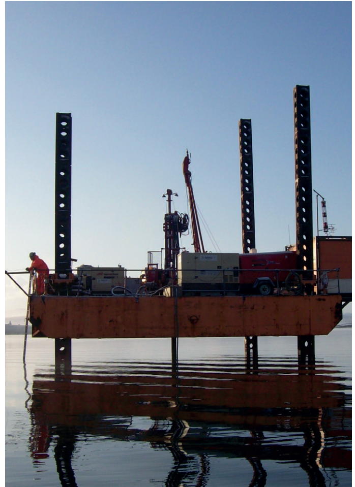
A vessel similar to this jack-up barge, with drilling equipment on board, will be used in the Deben Estuary.
