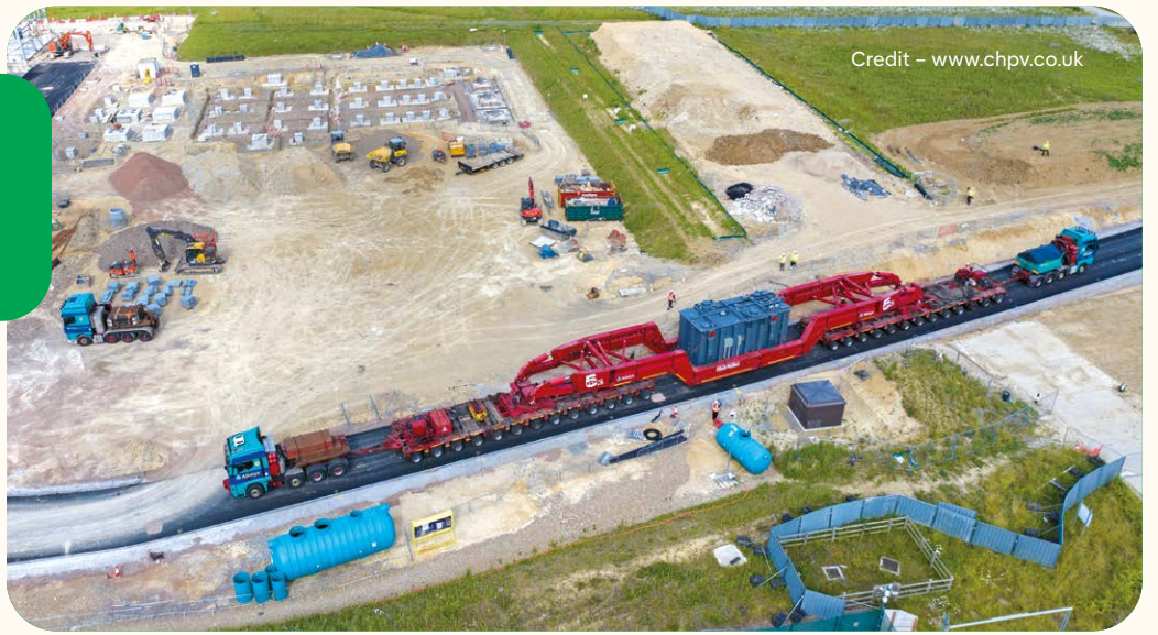
One of the four transformer units arrives at our Bramford site in June
