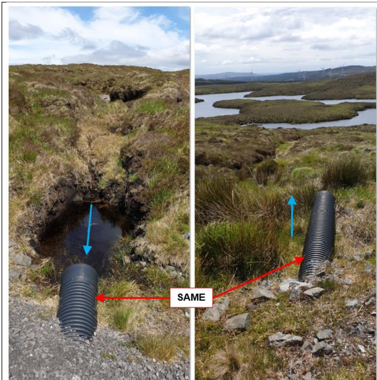
Example of Track Culverts and Drainage. Receiving surface water runoff from enhanced natural drainage channels and discharging to natural drainage channels on the downgradient side of the existing trackway.
