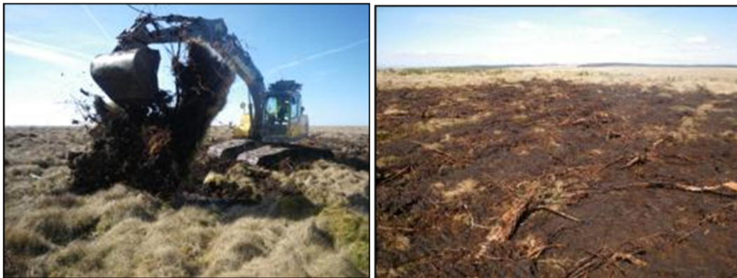
Photographs 1 and 2: Left (1) – excavator flipping an excavated tree stump. Right (2) – finished area after cross-tracking to smooth the ground surface.
