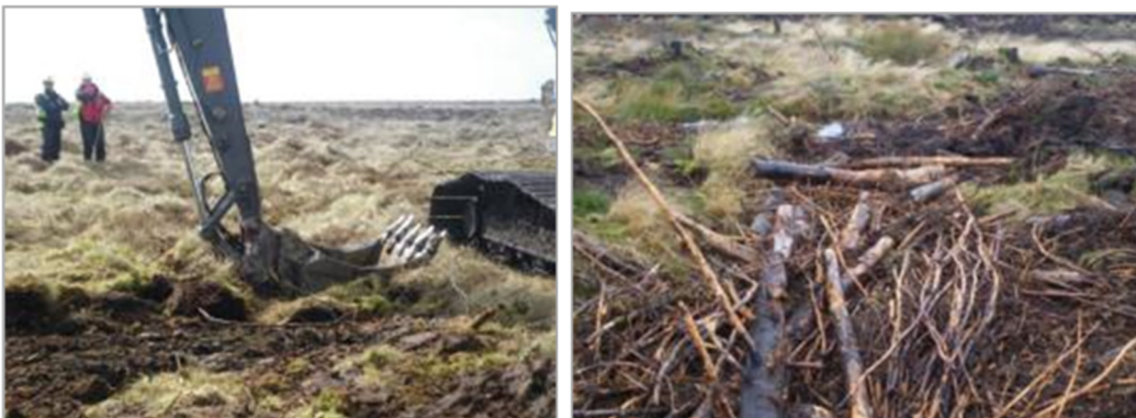
Photographs 3 and 4: Left (3) – excavator compacting material into a drain. Right (4) – drain infilled with forest brush.
